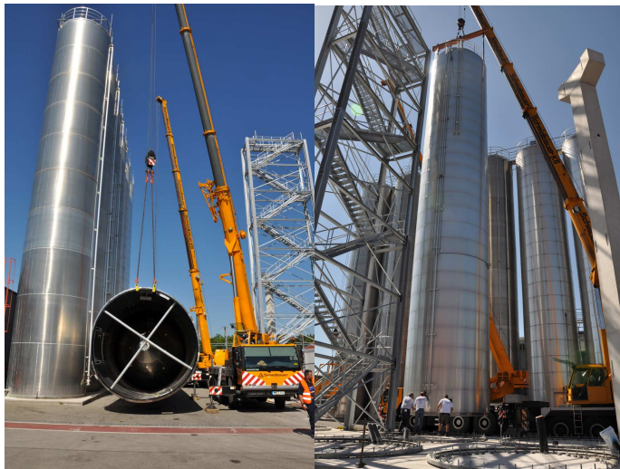
Construction of the new silo facility at the Salamander plant in Türkheim.
